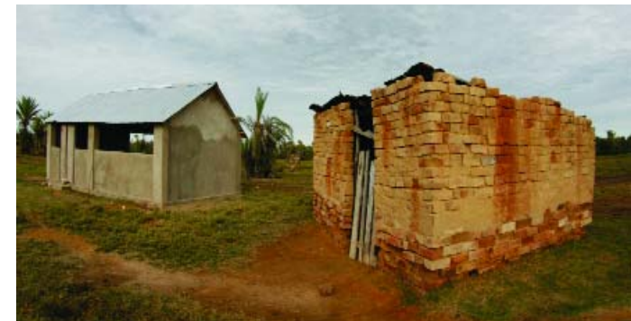
The new canteen and the existing kitchen - the next renovation project in the Ankoranga community action plan.
